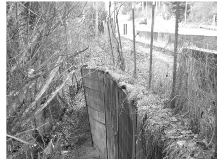
View of the challenged retaining wall with Oak Bay Road at upper right.
